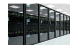
High heat density data center
