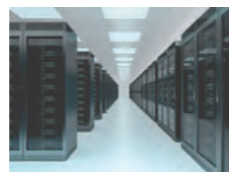
High heat density data machine room
