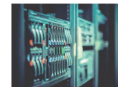
Container data center
