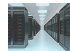
High heat density data machine room
